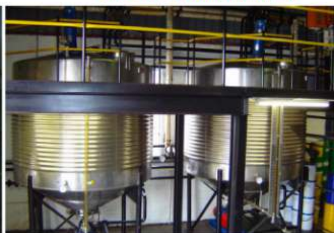
Processing Unit (Reactor)
